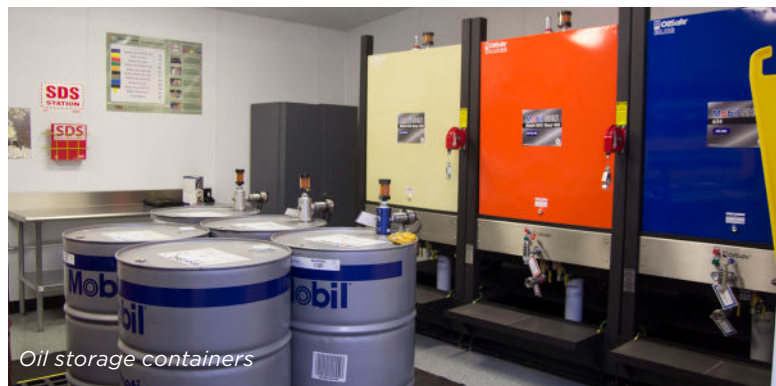
Top-up containers and grease gun storage
