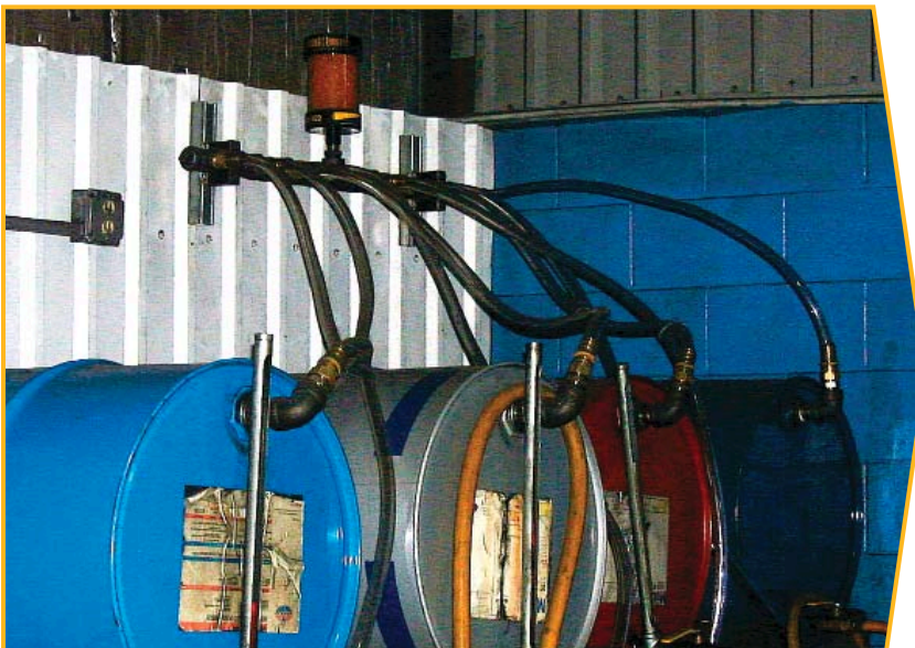
Eight Lubrication Drums Vented Through One Air Sentry® Breather
