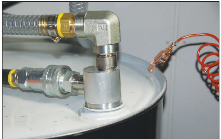
FIGURE 2: Static Discharge Grounding Wire
