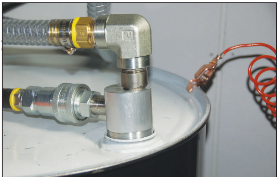
FIGURE 2: Static Discharge Grounding Wire
